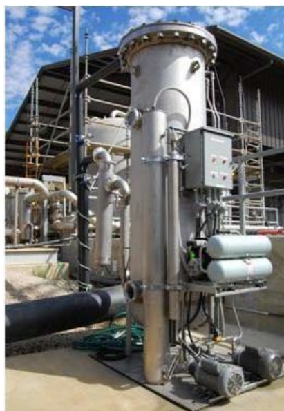
Figure 6. Nrgtek 100-SCFM Siloxane Removal System
